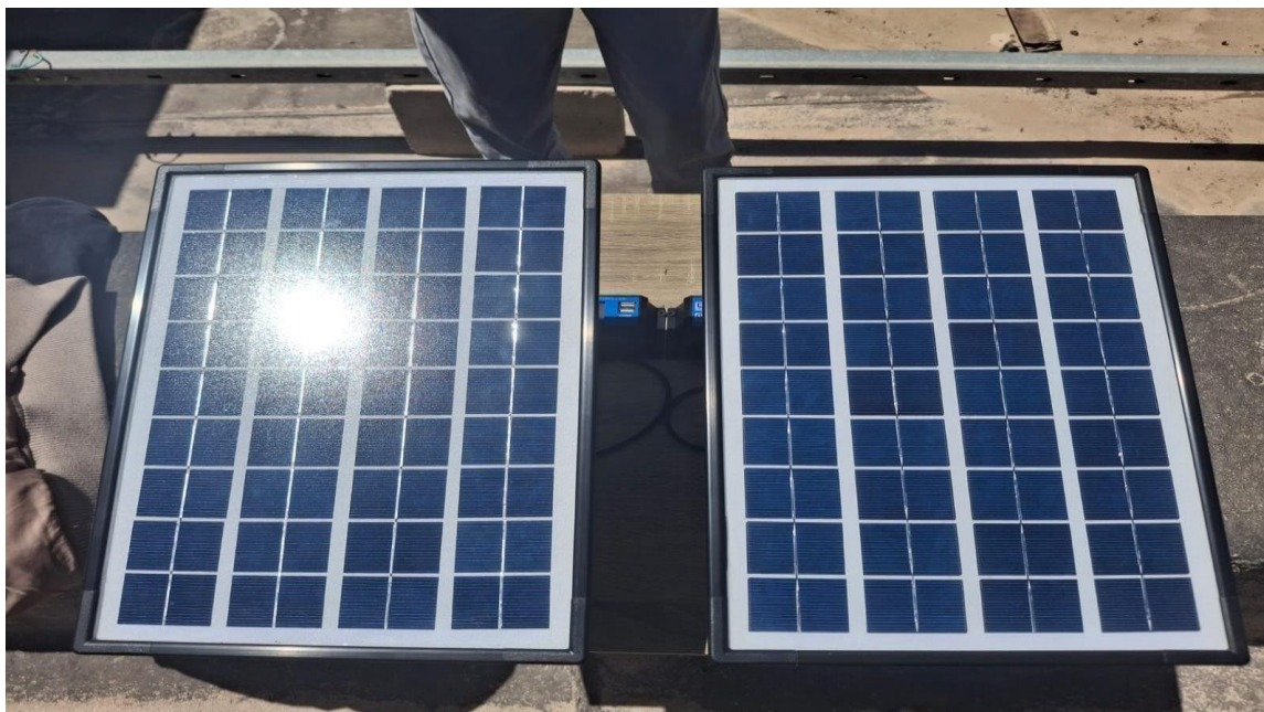
Figure 3.1 Two Identical PV Panels
