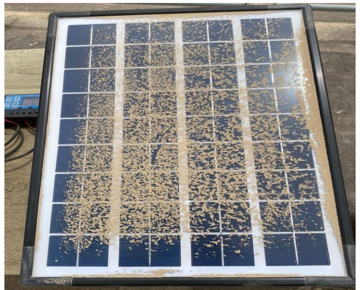
Figure 4.8 Uncoated panel after 24-hours
